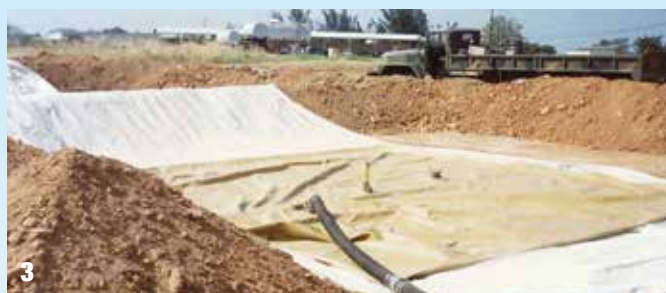
(1) A 528th SOSB refueling team used this 350 gallon-per-minute fuel pump at Fort Sherman, Panama, during a short deployment in mid-1989. The pump was later moved to Howard AFB and used during Operation JUST CAUSE. (2) Soldiers connect 4-inch hoses to the 10,000 gallon collapsible fuel bags. The bags are emplaced with the help of U.S. Army Engineers, who built protective berms around the site. (3) Once emplaced, the large fuel bags were ready to fill. The 528th SOSB FARP at Howard AFB used four of these bags during Operation JUST CAUSE.
