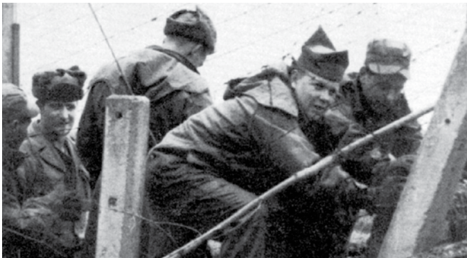
4th MRBC Rigger CPLs Bob Adams and Bill Keenan with others install fencing to prevent sabotage.
