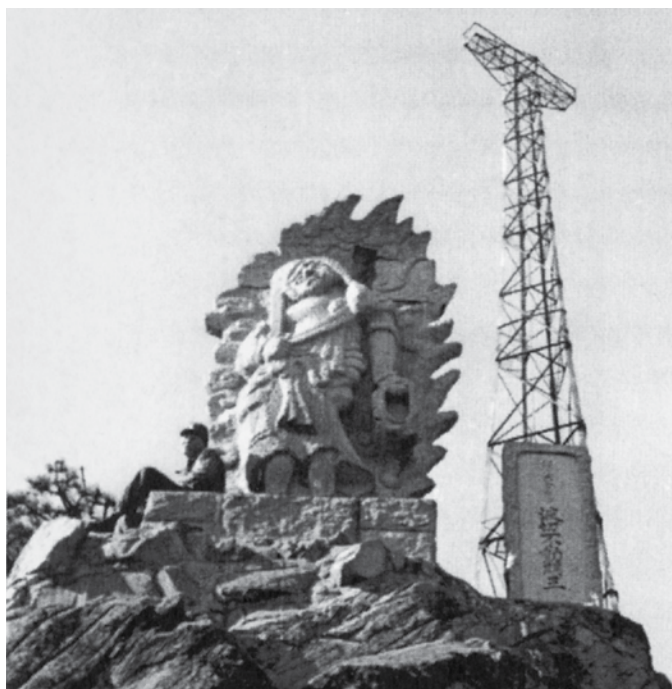
The 4 th MRBC antenna riggers installed a new double-doublet (T-bar) mast atop the Radio Seoul antenna to improve reception quality from Radio Pusan .
