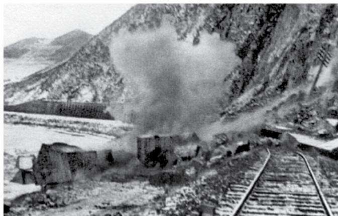
Cutting rail and rubbleing the entrances of railroad tunnels were UDT nuisance targets. Collapsing railroad bridges disrupted traffic for weeks.
