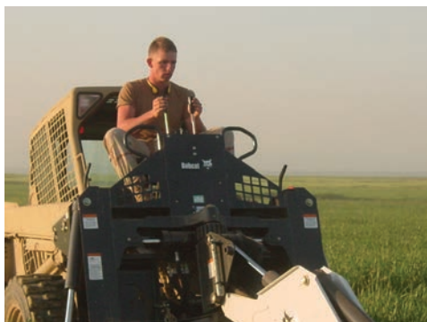
Figure 7.23 528th SOSB's Bobcat. Troops of the 528th Support Battalion used the Bobcat loader to great advantage in the construction of Camp Loki.
