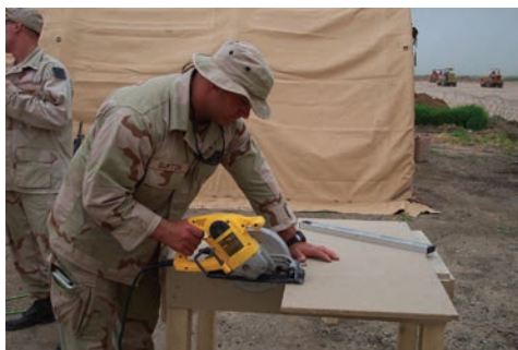
Figure 7.22 Construction skills. The construction of facilities at the camp tested the skills and ingenuity of everyone involved in the establishment of the camp.
